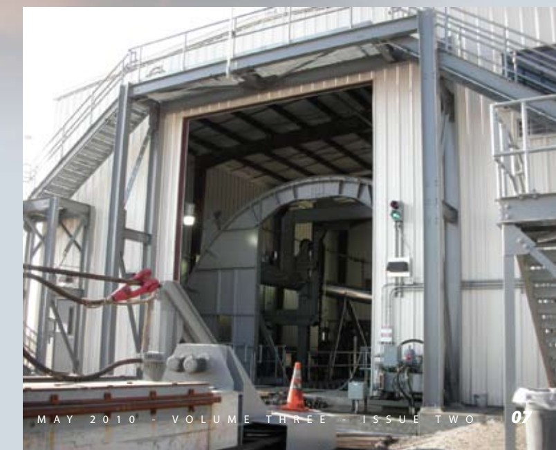
The rotary dump system is designed to flip each railcar upside down to unload the coal
