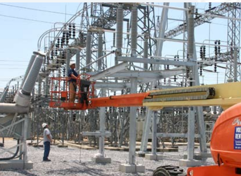
A contractor crew from H & H Construction, Inc. makes final adjustments to the 161kV switches at the Moselle switchyard
