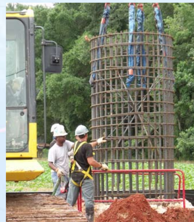
Tower foundations use steel to strengthen the concrete poured into the piers
