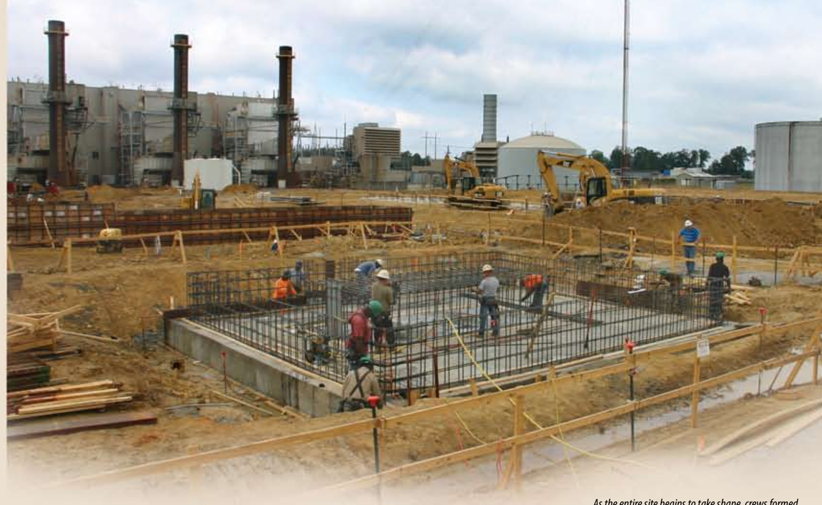
As the entire site begins to take shape, crews formed foundations for the step-up transformers (above, foreground) and for the Unit 2 combustion turbine-generator (photo below)
