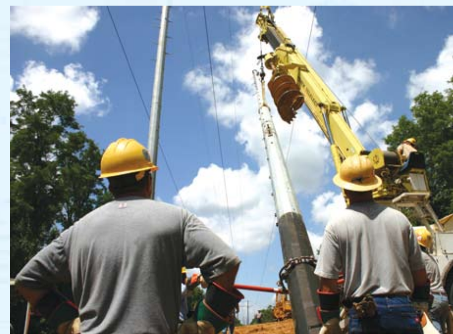
On a project last summer on Line 515 near Lorman, crews used steel poles to replace wood poles that had deteriorated.
